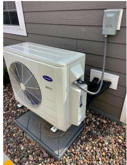
Heat pumps are a sustainable heating option, but work best where buildings have first been properly insulated. Photo credit: Wikipedia.
